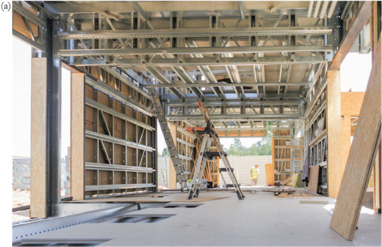
Figure 57. Prototype construction, (a,d) ground floor structure, (b,c) infrastructure through structure, (e) vapor barrier, (f) exhaustion through structure, (g,i,j) stairs, (h) first floor structure (cont.)
