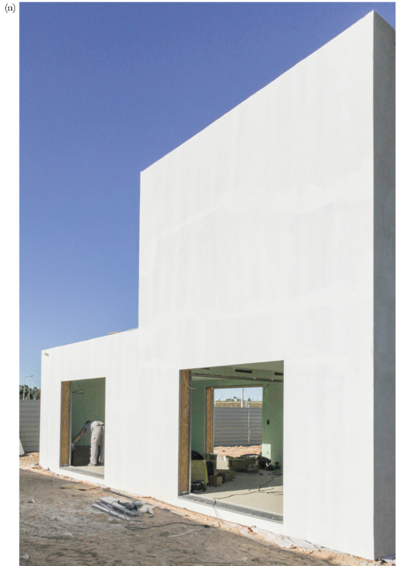
Figure 57 (cont). Prototype construction, (k) OSB over structure, (m) finishing external layer (l,n) concluded raw elements.
